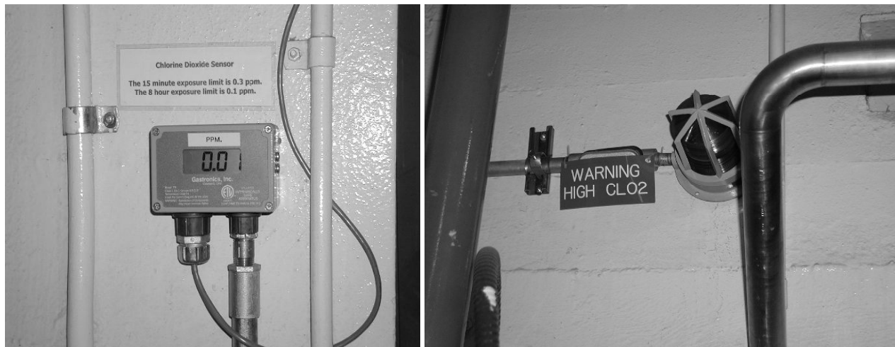
Figure 2. Chlorine dioxide monitor (left) and chlorine dioxide alarm (right).
